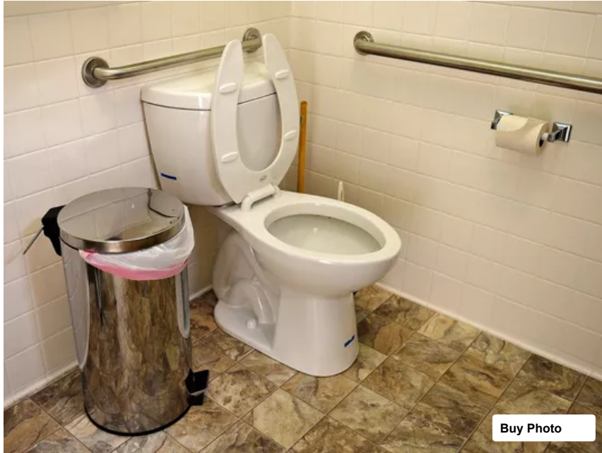
Paul Hegland and Bob Mann installed highly efficient toilets in the common house at River Rock Commons Cohousing Community. The new toilets use .8 gallons per flush, about half the water used by the previous toilets. (Photo: Valerie Mosley/The Coloradoan)
